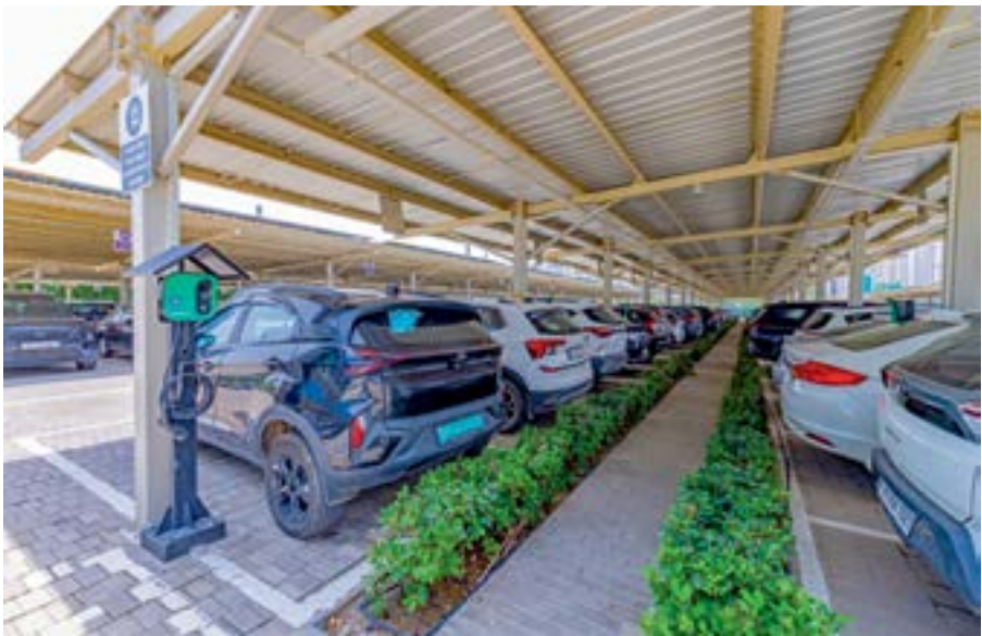
EV charging zones at DLF Offices
