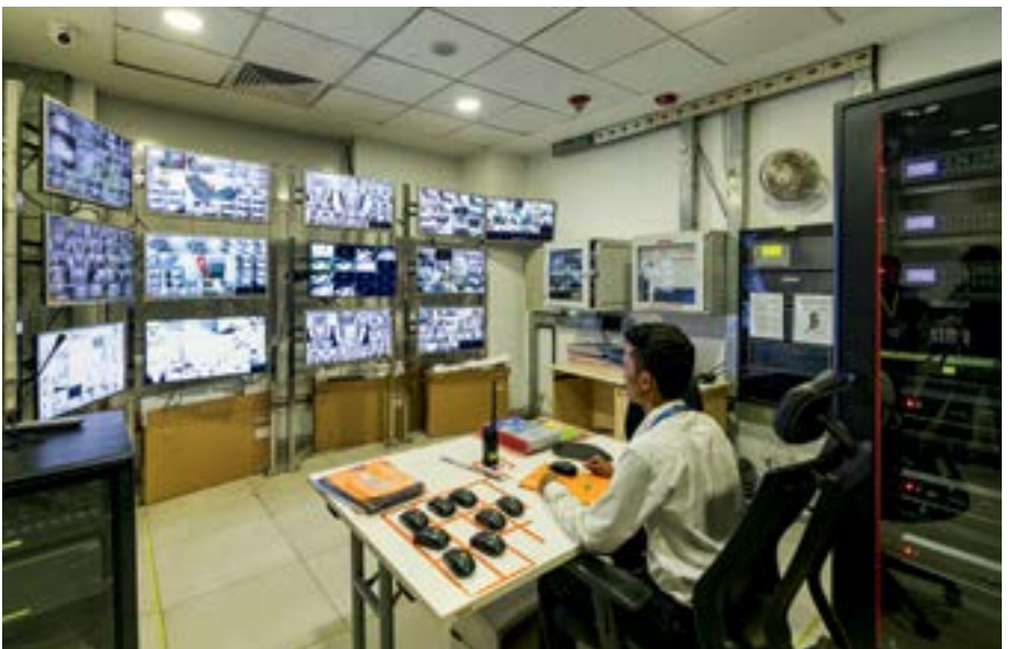
CCTV Monitoring at Cyber City, Chennai
