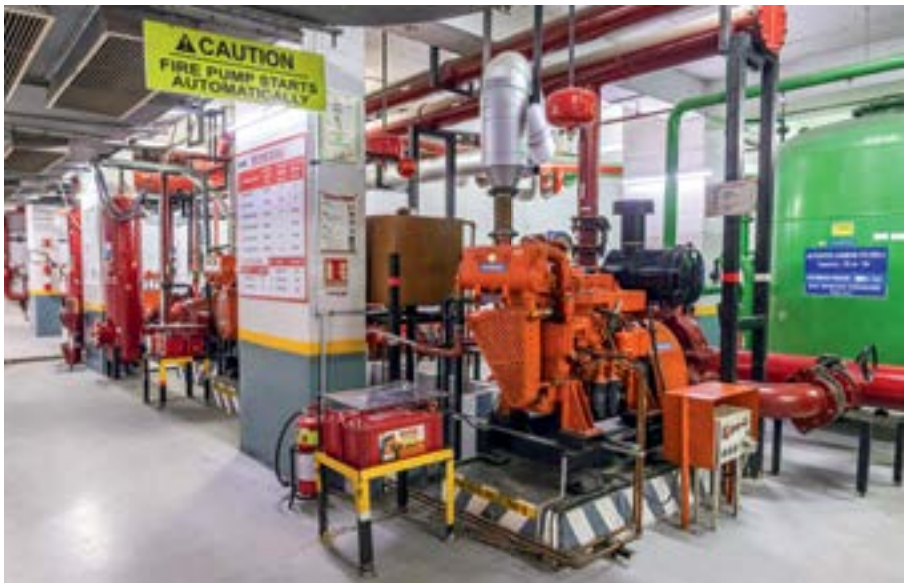
Fire Pumps at our buildings
