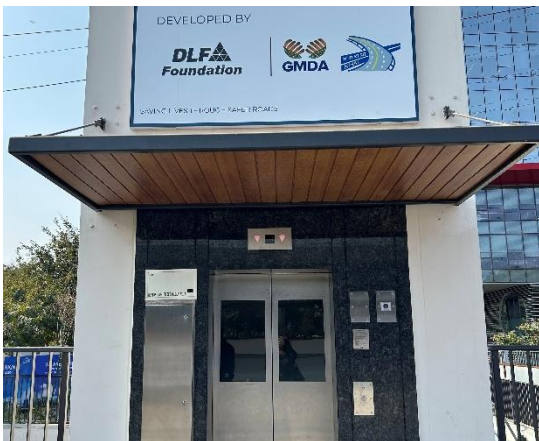
Lift installed at Subway-B
