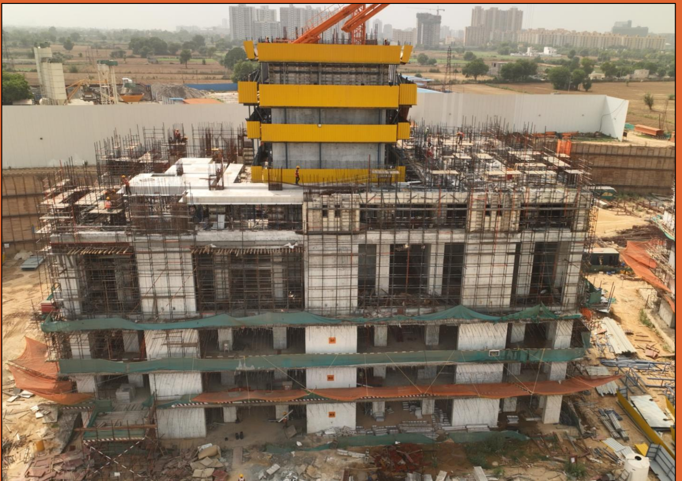
Tower F 3 rd Floor Core wall Casted ; 1 st Floor Slab Casting WIP
