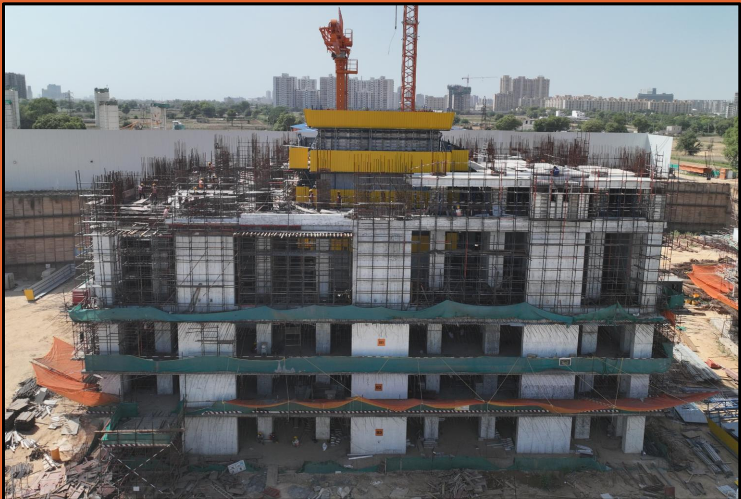
Tower F 3 rd Floor Core wall Casted ; 1 st Floor column casting work in progress
