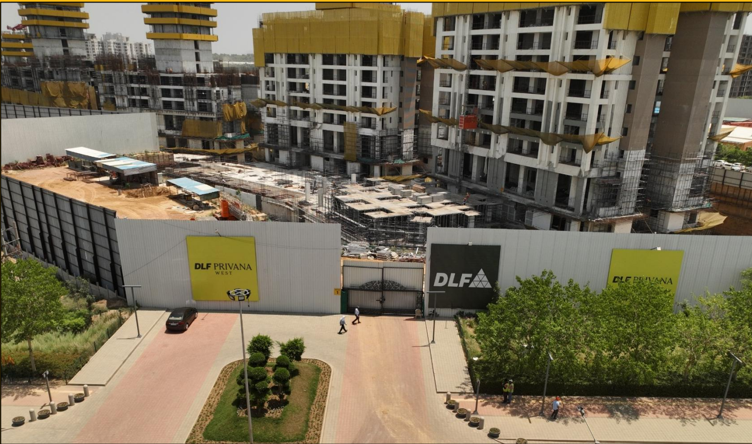
MAIN ENTRY GATE
