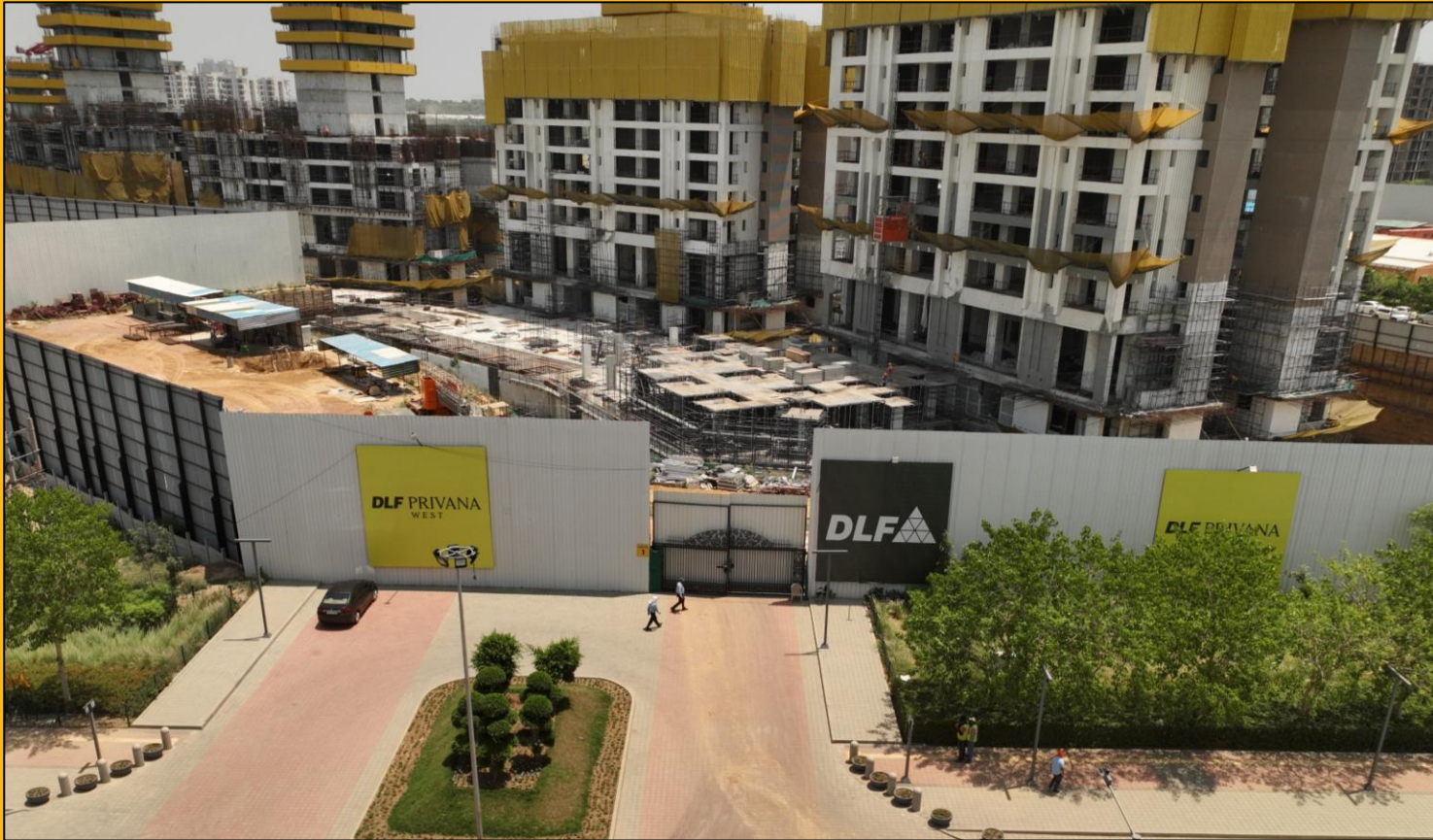
MAIN ENTRY GATE
