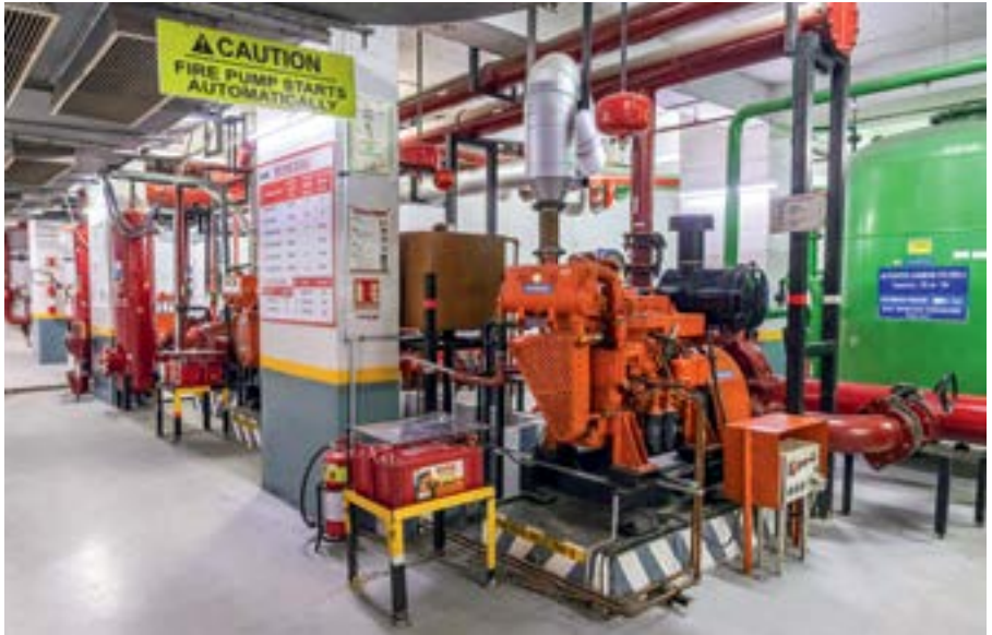
Fire Pumps at our buildings
