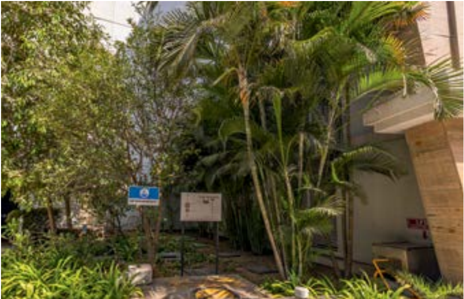
Rainwater Harvesting pits at DLF Cyber City, Hyderabad
