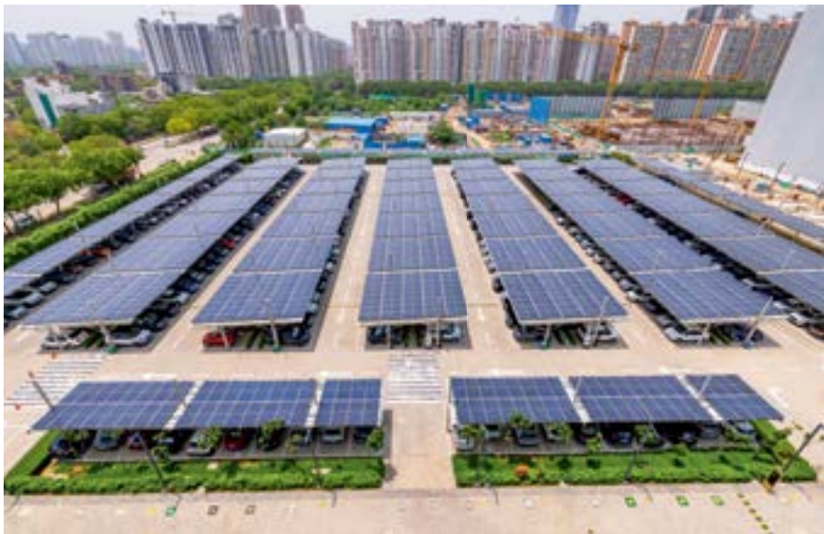
Solar Panels installed at DLF Techpark, Noida
