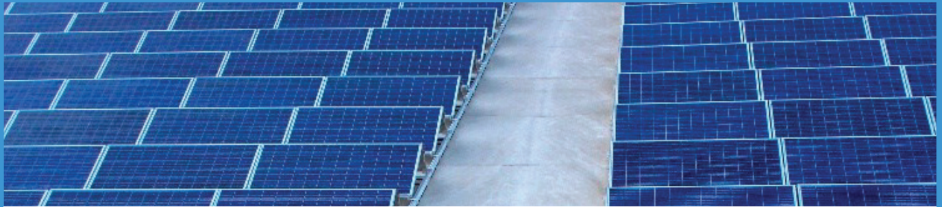
Solar Plants of capacity 2.68 MW are installed on the roof top across DLF Rental business buildings. We are working toward further enhancement of capacity of solar plant.
